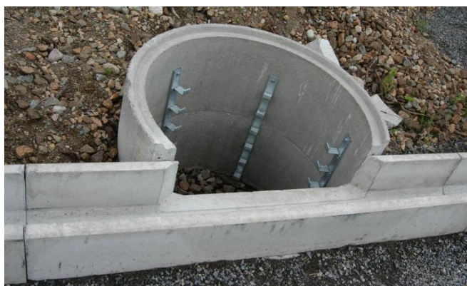
Well for wires.
